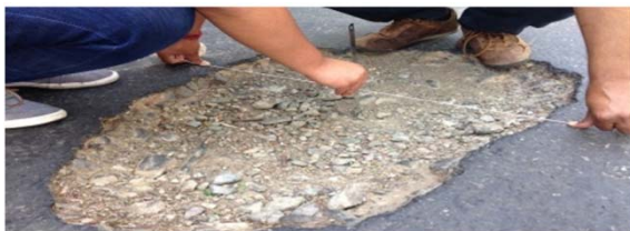
Fig. 2: Showing Depth of Pothole
